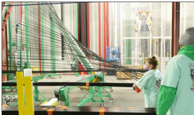
Figure 3. Personnel at the Garden City plant monitor the coated extrusions as they come off the new CUBE vertical powder coating line.
